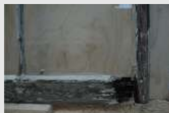
Before our work this window appears beyond repair
